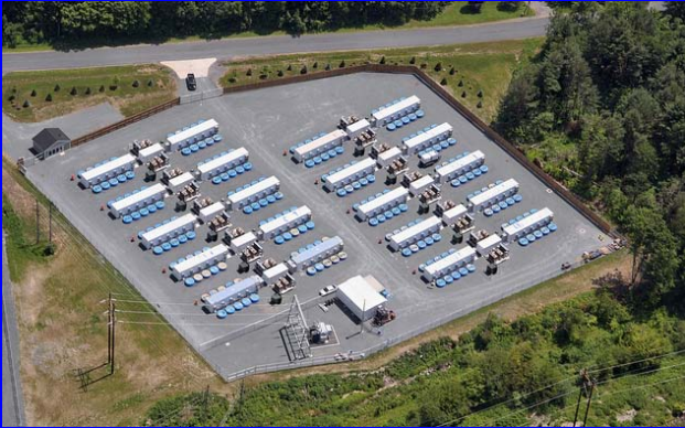
20MW Flywheel Storage for Frequency Regulation - NY
